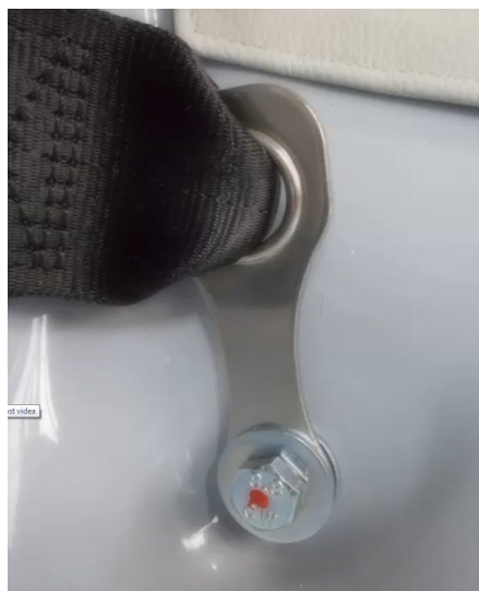
Figure 53-003 Safety harnesses attachment point on the cabin floor
